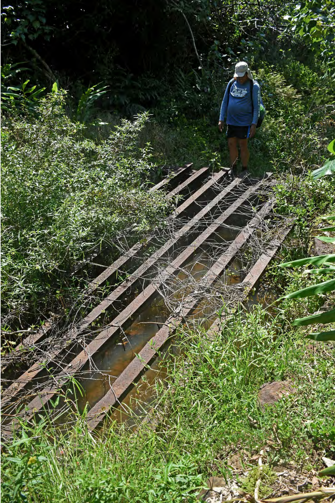
Fig. 17. Station 2, Lowrie Ditch at the Long Strainer and intake L-15, along an eastern tributary to Honopou Stream. The ditch in this area is not flowing, and is heavily overgrown with weeds.
