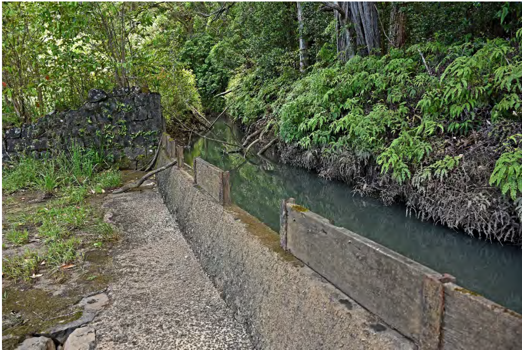
Fig. 16. Spillway along New Hamakua Ditch, emptying into a tributary to upper Huelo Stream northeast of New Hamakua Ditch intake N-17a. Note the fallen trees in the ditch, which is not flowing at this point, and missing flash boards along the spillway, indicative of disrepair.
