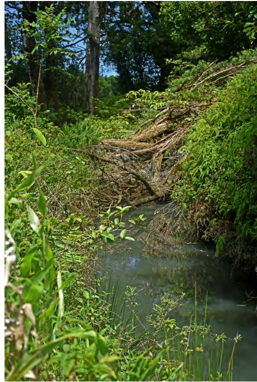
Fig. 8. New Hamakua Ditch east of Intake NH-17a, showing significant blockage by fallen trees.
